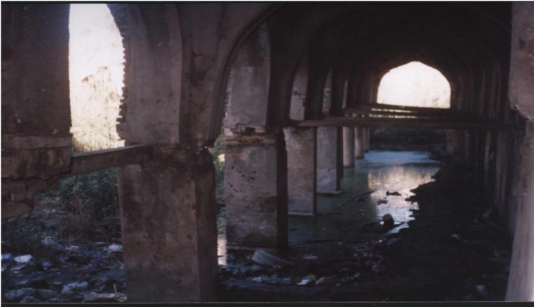
Figure 2-20: Deteriorating conditions of Historical sites
